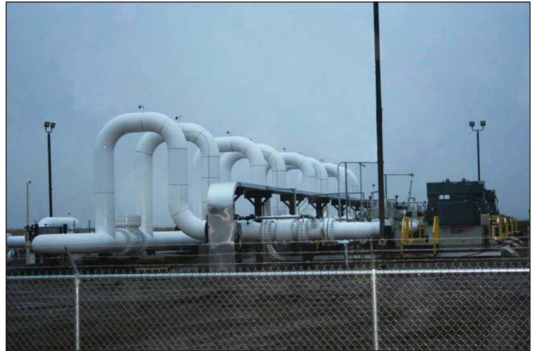
A pumping station for Keystone 1 in eastern North Dakota.
